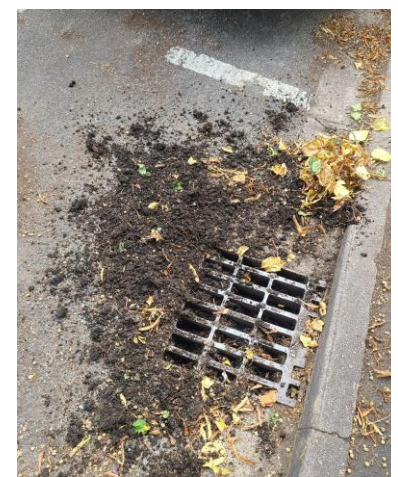
Gullies/drains filled with detritus
